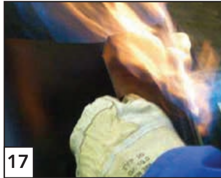
17 Warm one end of the adhesive side of the closure patch with a gas flame. Position the warmed side of the closure patch over the exposed edge of the sleeve.
